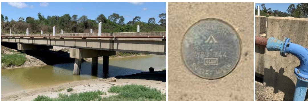
Plate 10-1 Ogmores Road Bridge Crossing at Styx River and Permanent Survey Marker [Source: WRM Water & Environment, October 2019]
